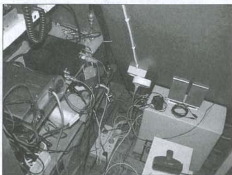
Fig. 5 Installation in the cottage about 60 meter from the antennas with the radio, power supply, computer and Internet connection
